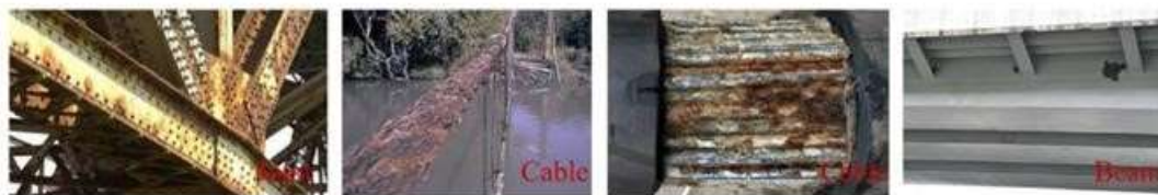
Fig 2.2 Typical corrosion of steel bridge (source: Chuang Cui 2024)
