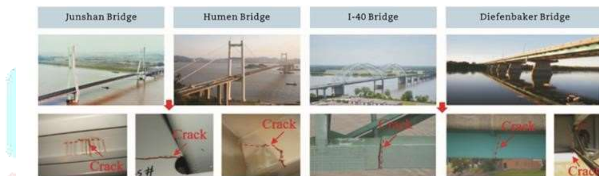
Fig 2.1 Typical fatigue cracks in different bridge types (source: Chuang Cui 2024)
